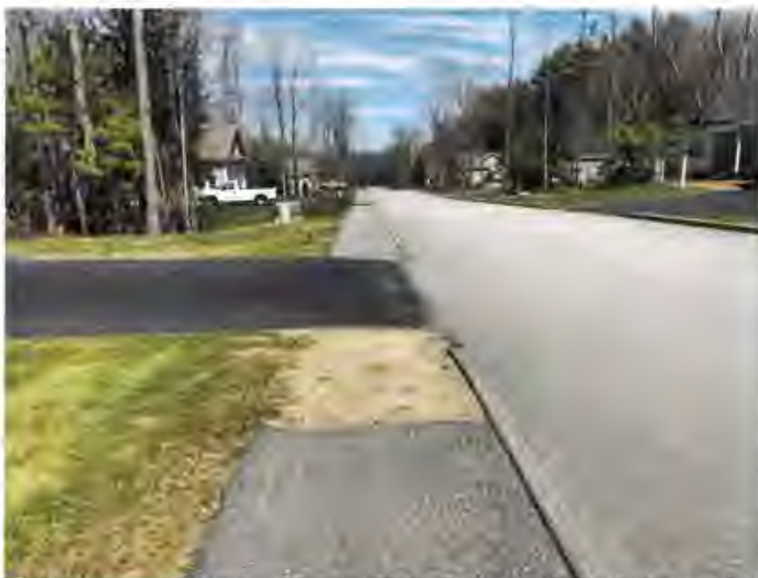
Photo 2: Sidewalk Incomplete Along Neptune Road (Photo Taken by Jaime Wallace, PE Dated 4/27/2021)
