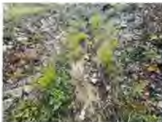
Erosion in armored scale to Infiltration Basin #1.
