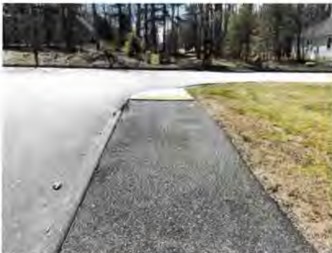
Photo 1: Alignment Issue with Detectable Warning Device Along Neptune Road (Photo Taken by Jaime Wallace, PE Dated 4/27/2021)
