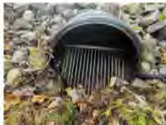
30" outlet to Infiltration Basin #1.
