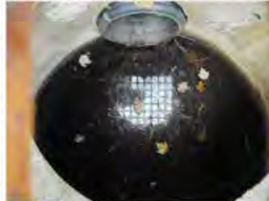
Typical CB sump (CB#3).
