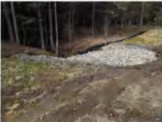
Photo 3 – Level Lip Spreader Beachmont Subdivision - Old Orchard Beach, ME Taken by Steve Blais, 5/12/13
