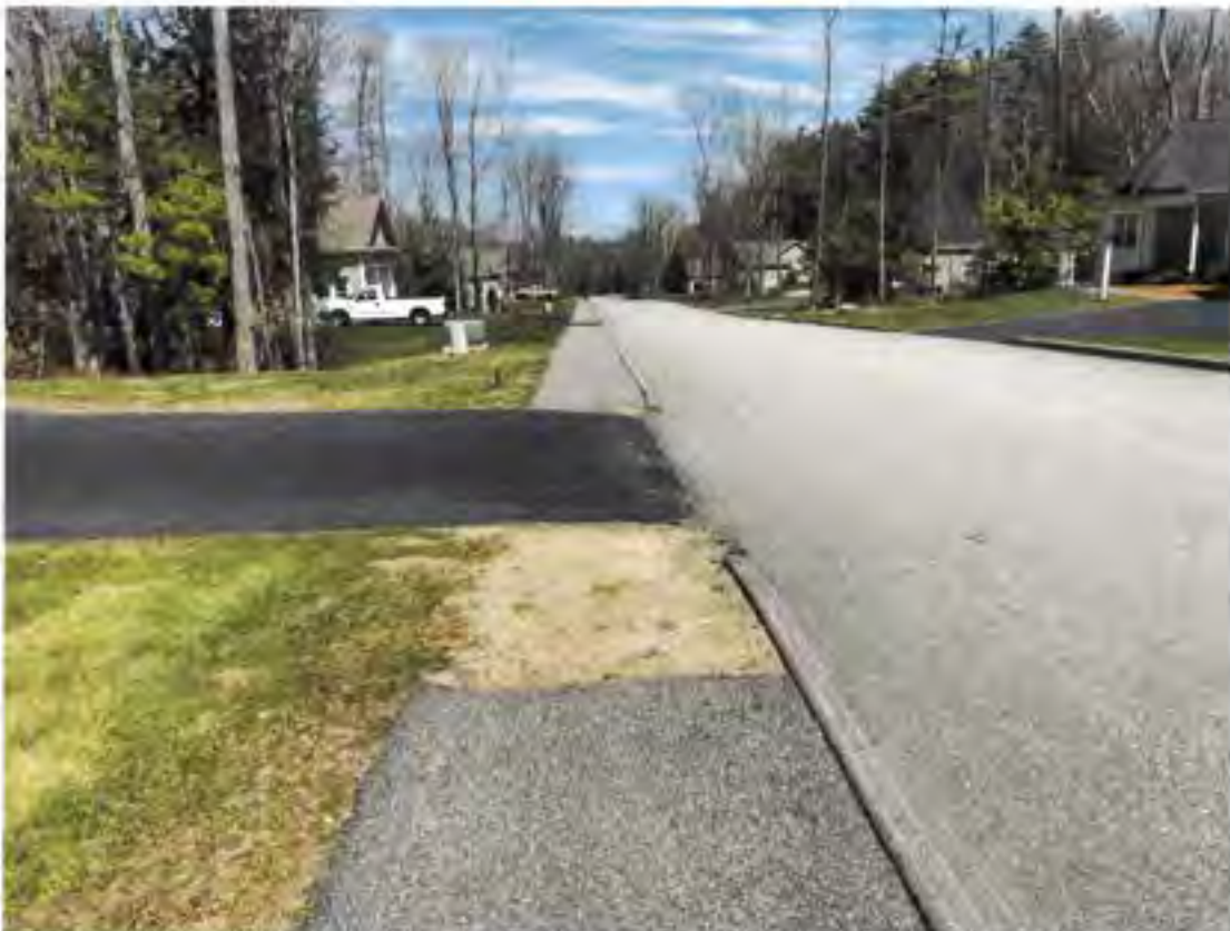
Photo 2: Sidewalk Incomplete Along Neptune Road (Photo Taken by Jaime Wallace, PE Dated 4/27/2021)
