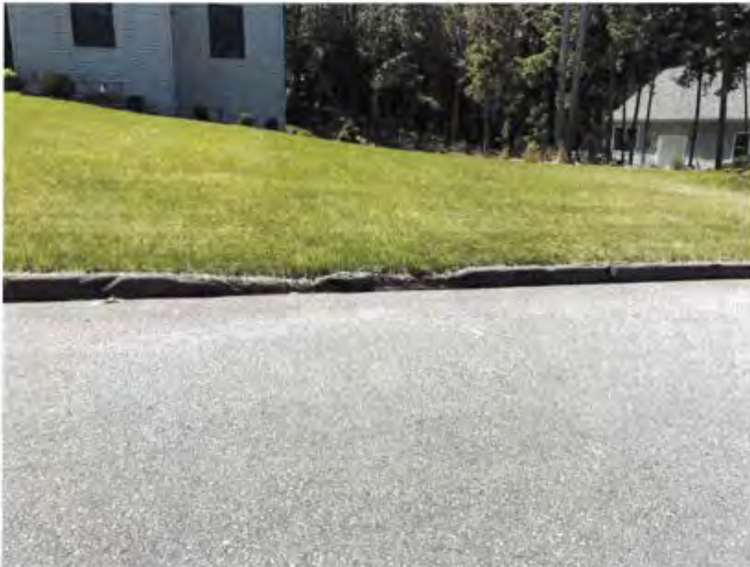
Photo 3: Damaged Curbing Along Dolphin Ave. (Photo Taken by Jaime Wallace, PE Dated 4/27/2021)
