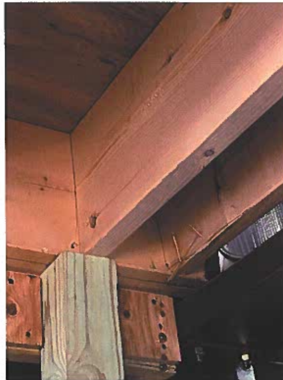
Photo 2: Inadequate Beam to Post Connection
