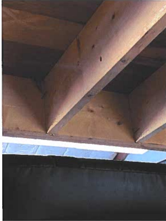
Photo 1: Inadequate Face Nailing Connection
