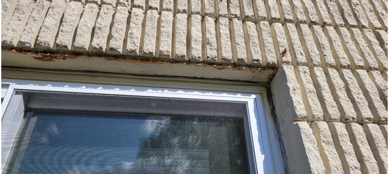
The steel lintel above window has begun to corrode. No signs of any existing flashing along top of lintel.
