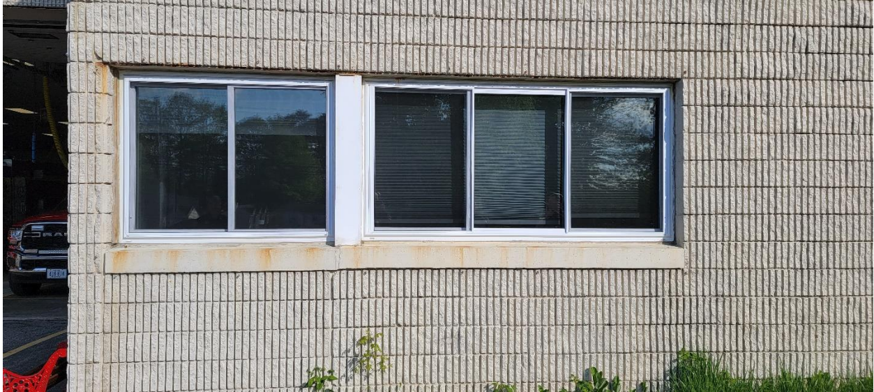
Window and corner of building where water has been entering inside the building.
